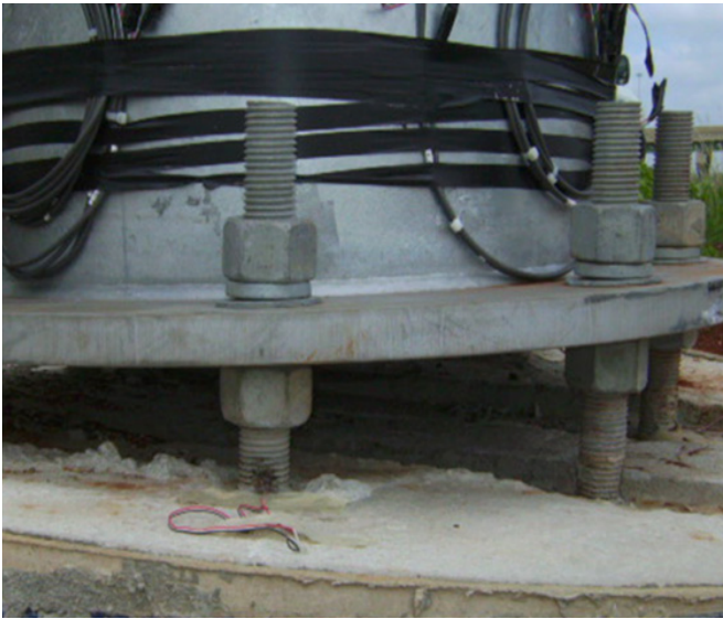
Sign base with anchor bolt clearance discrepancy.
